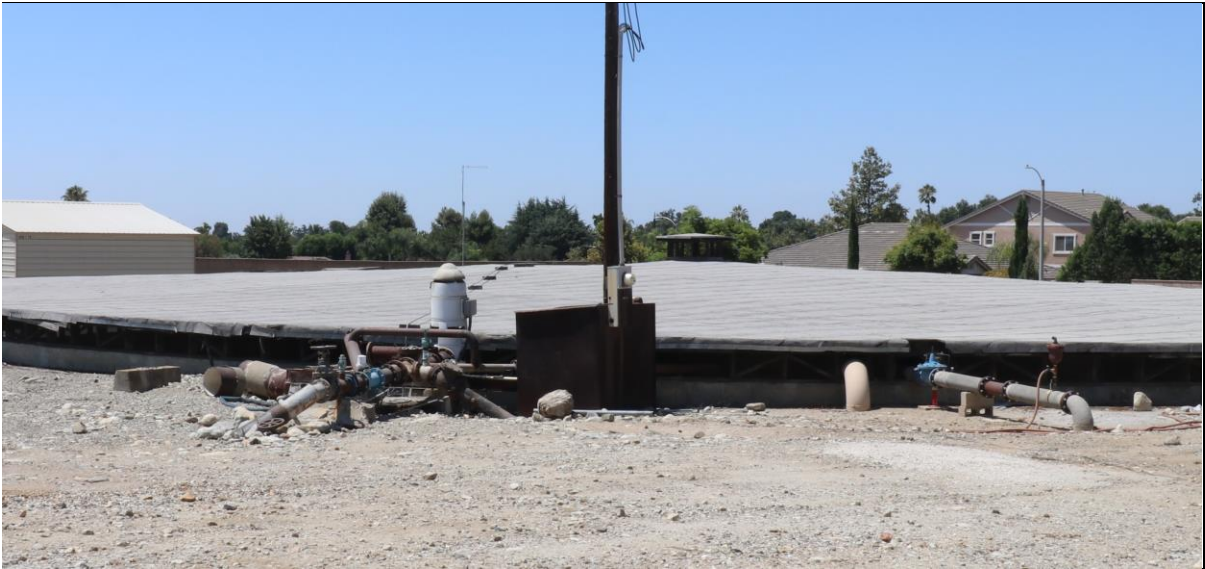
Photo 2: Equipment on the northeast side of the reservoir, view southwest (8/6/24).
